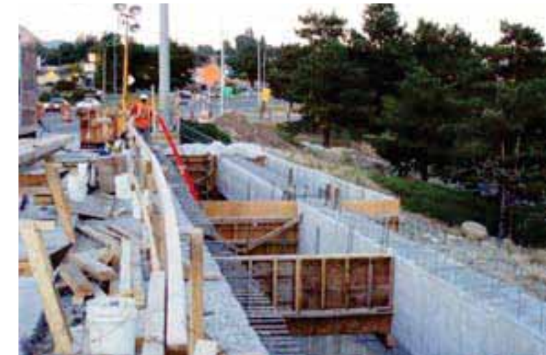
Washington State DOT adds a cantilevered bicycle and pedestrian structure to the existing Sellar Bridge connecting Wenatchee and East Wenatchee. Image | Flickr.com (wsdot)
