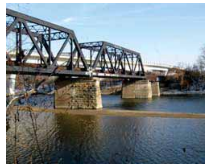
The rail bridge just south of SR 26 as seen from West Lafayette. Image | Stanton Lambert
